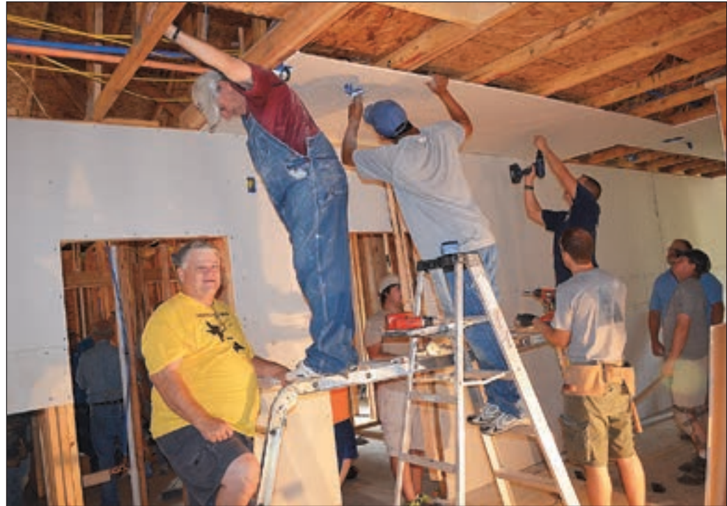
▲ Robbie Caldwell (on left), pastor of New Harmony Baptist Church, and a group of volunteers from his church install sheetrock in the new JC residence hall.
