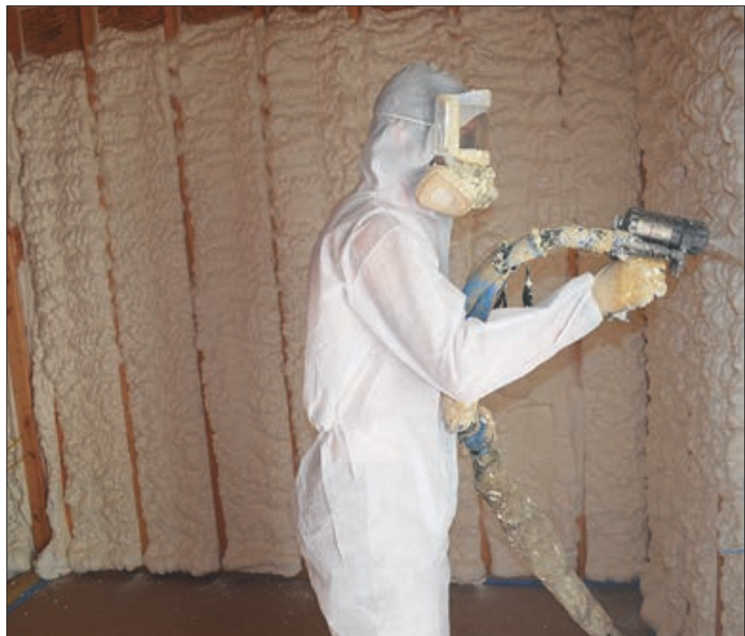
▲ JC alumnus Tommy Cockerell of D & D Insulation and Foam in Fairfield sprays insulation from floor to ceiling in the new residence hall.
